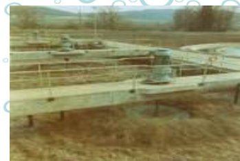
biological reactor with fixed surface aeration system.
