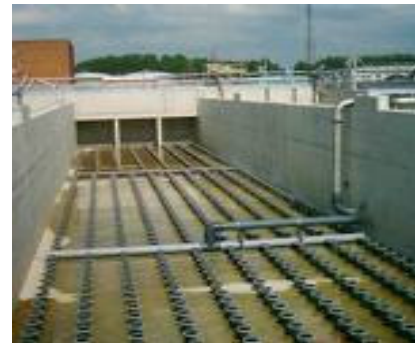
biological reactor with fine bubbles diffusers system.
